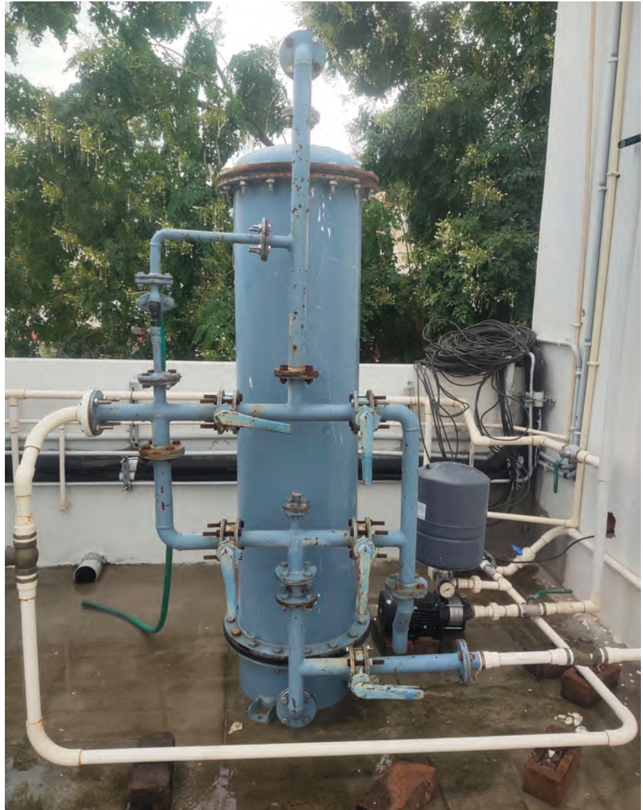
Commercial Water Treatment Plant by Aquality Water Solutions
