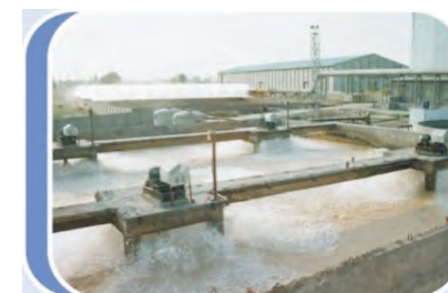
Effluent Treatment Plant
