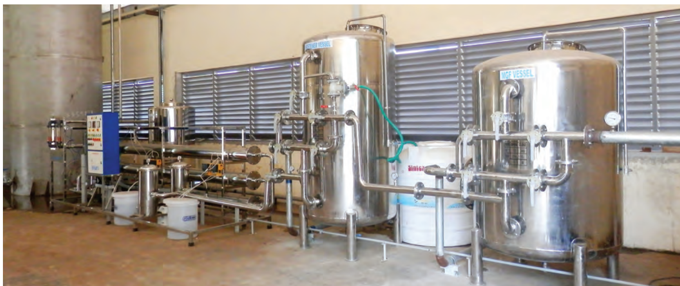
600 KLD Reverse Osmosis System for Boiler Feed
