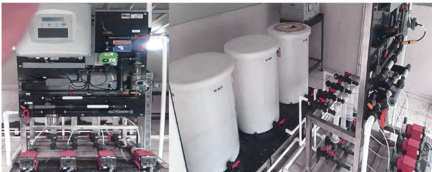
Images of Nalco's 3D TRASAR system installed
