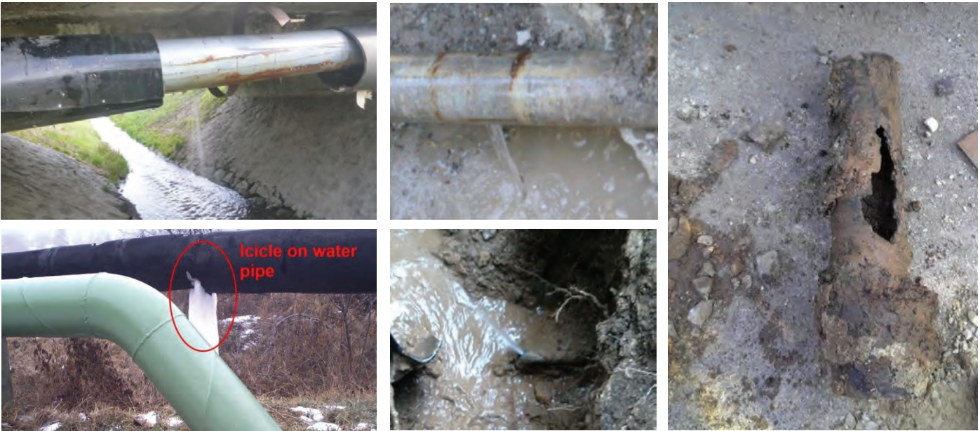
Figure 13: Photos of visible and invisible (hidden) leakages
