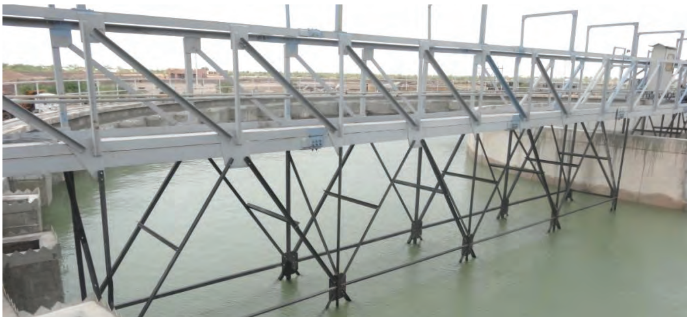
Water Treatment Plant at Pokhran, Rajasthan
