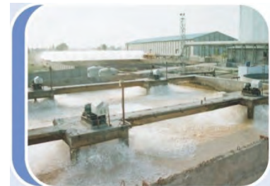
Effluent Treatment Plant
