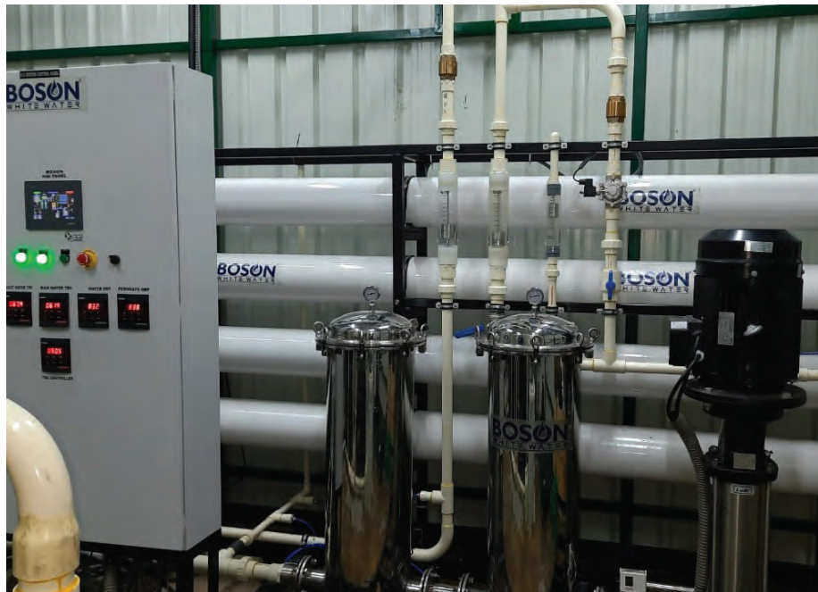
BOSON White Water System Installed at a commercial Mall
