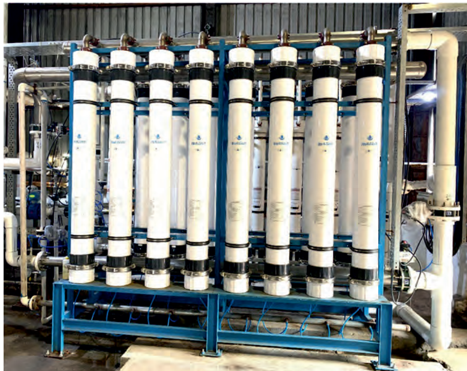
Figure 8: MOWS Ultra Klean UF train – Phase II condensate treatment, Sugar processing Unit, Nellikuppam, Tamilnadu.
